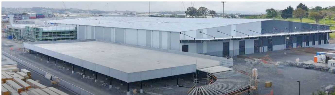
The new APC under construction in Auckland. It will feature 3D scanners to detect biosecurity threats.
