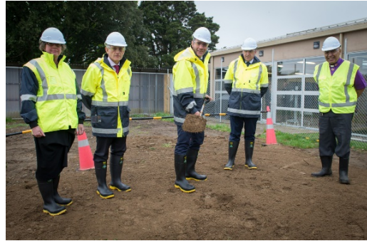
The Minister for Primary Industries turns the first sod. From left: Lyn Provost (Controller and Auditor-General), Martyn Dunne (Director-General, MPI), Hon Nathan Guy, Andrew Coleman (Chief Operations Officer, MPI), Bill Herbert (local Kaumātua)
