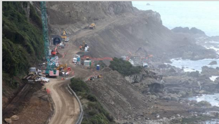
Ongoing cliff erosion and road works
